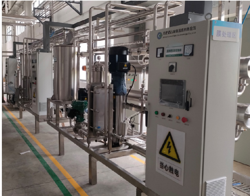
Figure 8. Reverse osmosis concentration equipment
