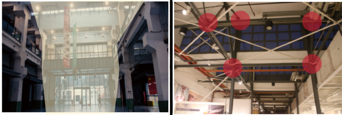
Figure 5. Reinforcement of internal atrium and steel structure node in phase II plant renovation (photographs by the author)
