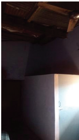
Figure 16. View of the newly added attached bathroom to bedroom; false ceiling done in bedroom.
