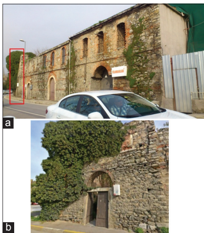
Figure 1. General view of the historic warehouse; (a) front view, (b) side view [4]
