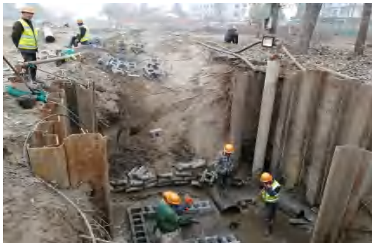
Figure 5. Pipe end misalignment
