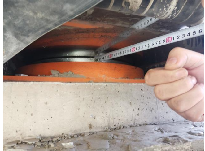
Figure 10. Longitudinal large pile number displacement of 1-2# support
