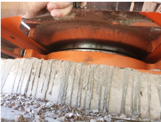
Figure 7. Longitudinal large pile number displacement of 1-1# support
