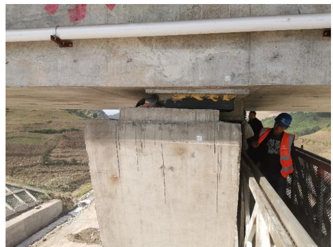
Figure 8. Longitudinal large pile number displacement of 1-1# support
