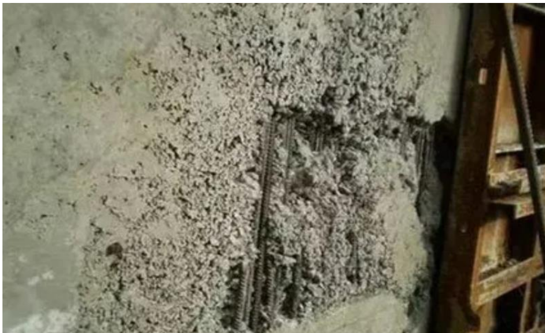
Figure 1. Denudation of the bridge surface
