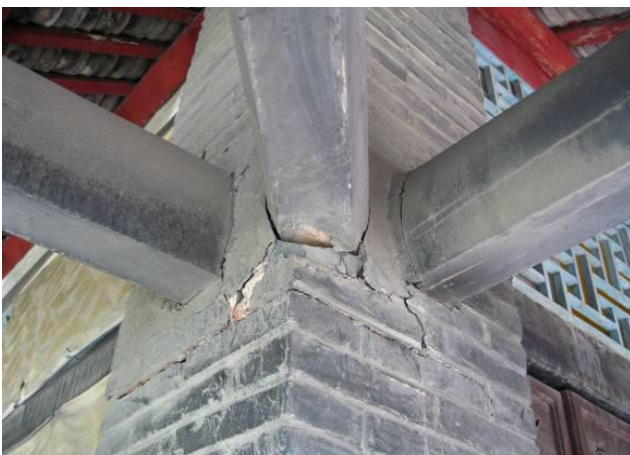
Figure 7. Cracks seen on the brick column of Yuhuang Hall after the earthquake
