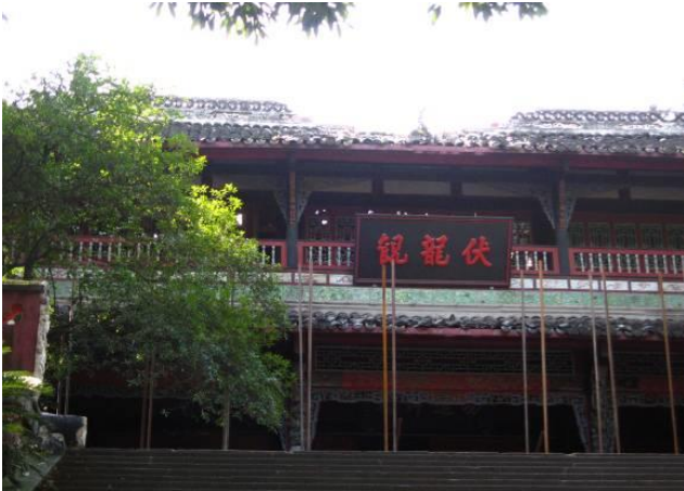
Figure 5. Front view of Fulong Taoist Temple after the earthquake
