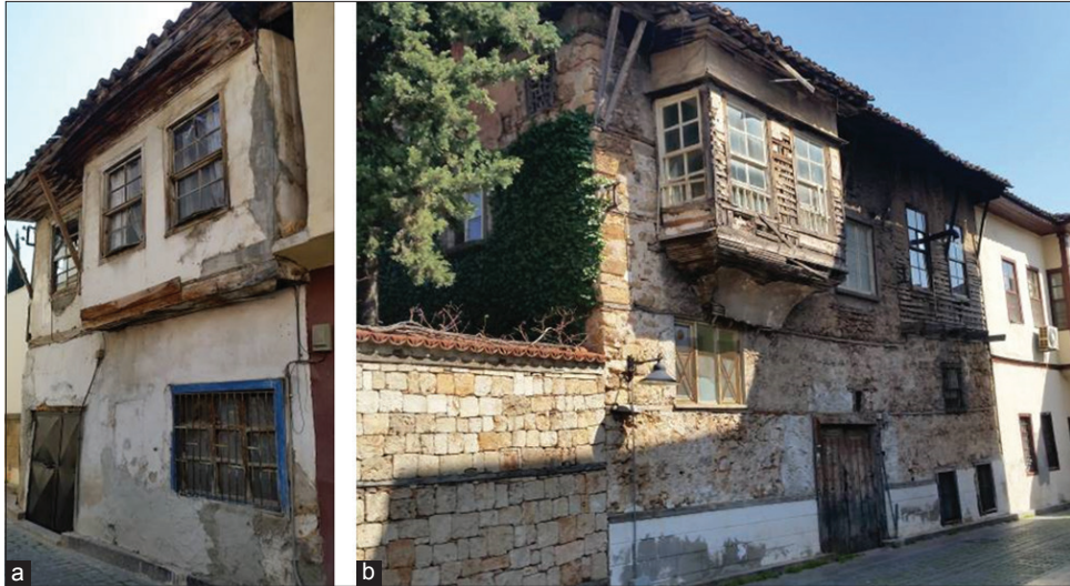
Figure 5. (a and b) Traditional buildings in the historical center of Antalya (Turkey)
