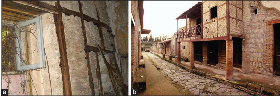
Figures 2. (a and b) Opus craticium: Particular of a wall (left), House of Frameworks in Herculaneum (right)
