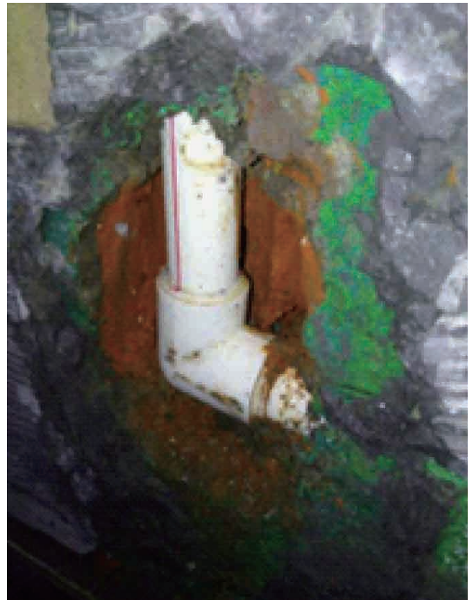
Figure 1. Leakage of underground pipelines
