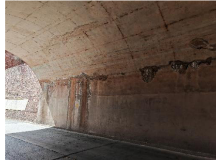
(b) Water seepage marks on the lining surface
