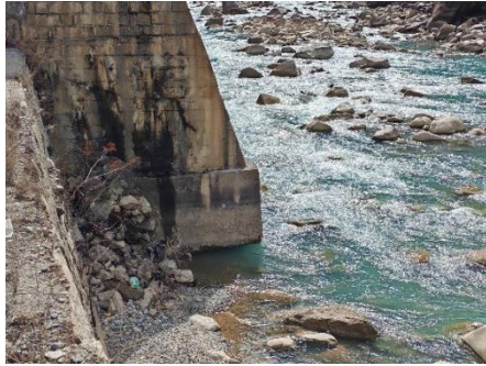
(a) The bottom of the foundation of the portal is hollowed out
