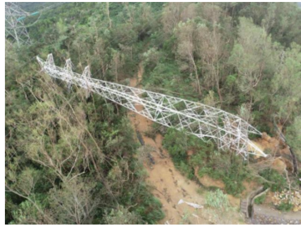
Figure 3. The tower foundation gave way
