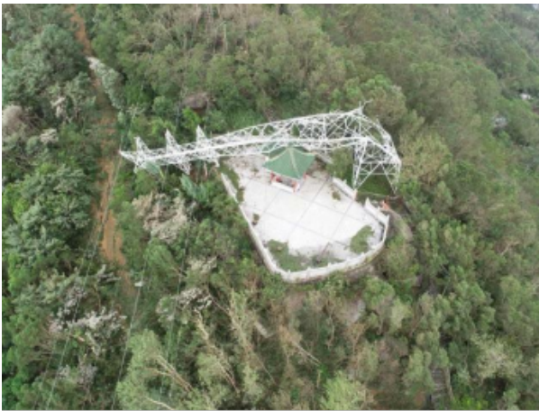
Figure 2. The tower body is bent
