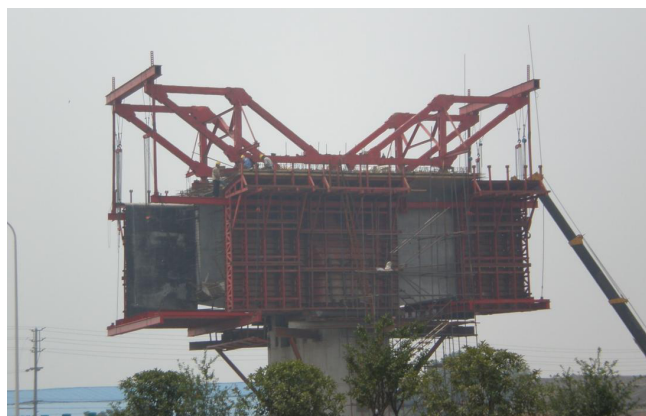
Figure 3. Photo of the installation work of the hanging basket at the construction site
