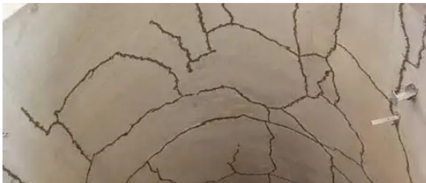
Figure 2. Secondary lining cracking in Jinfeng Tunnel
