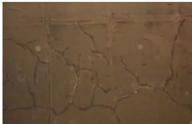
Figure 1. Reticulated cracks in the secondary lining
