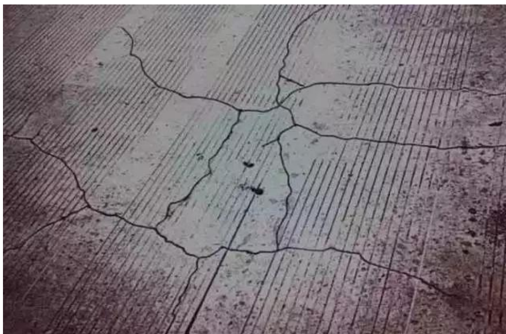
Figure 1. Cracking type of concrete crack
