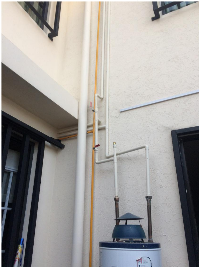
Figure 3. PVC used in pipes (photo: Silverio Hernández-Moreno, 2018).
