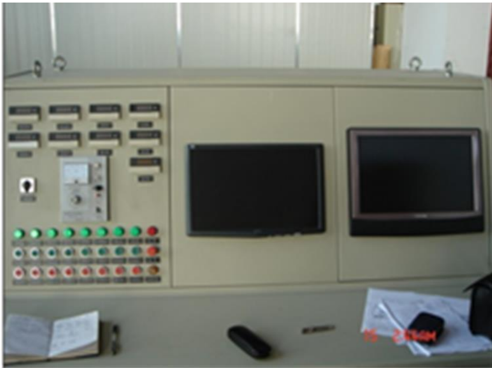
Figure 3. PLC control cabinet
