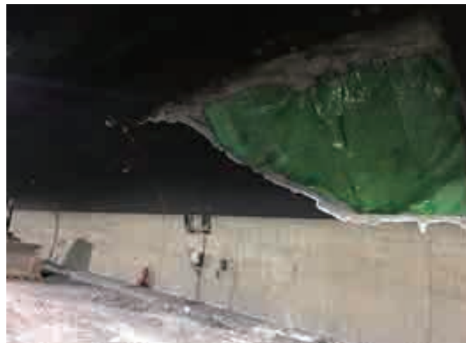
Figure 1. Partial exfoliation of the tunnel secondary lining
