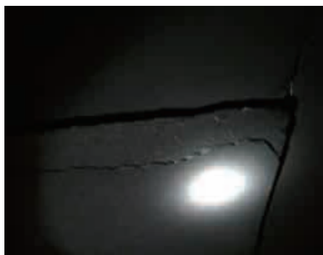
Figure 2. Faulting of slab ends on the secondary lining on the right side of vault of the k21+241 segments
