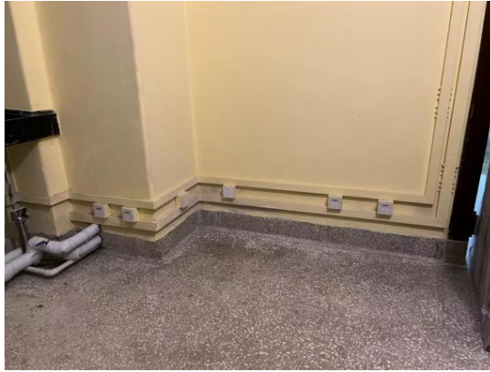
Figure 8. Surface mounted electrical circuit
